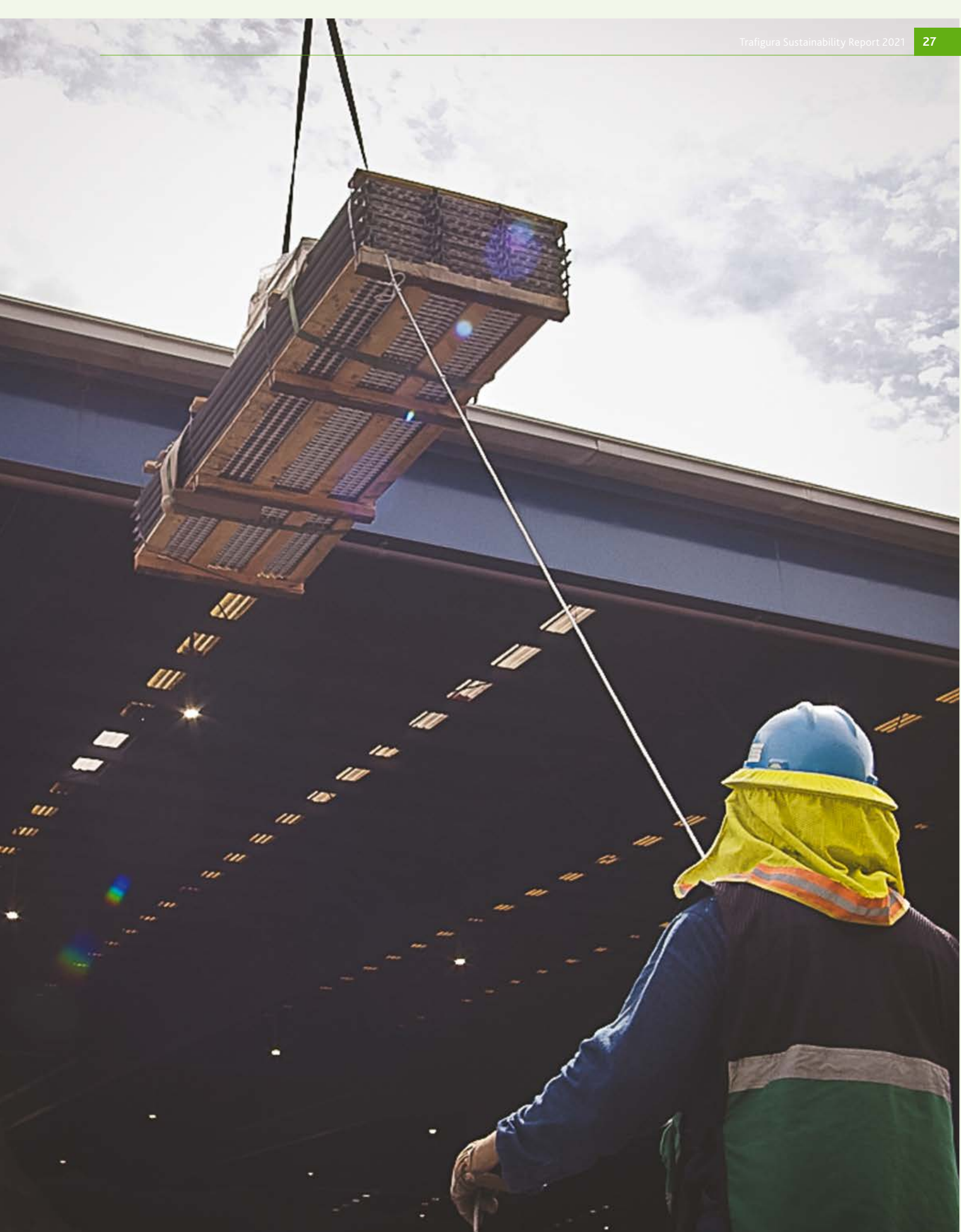
Installing the last of the 1,500 solar panels on the roof of the Impala Terminals building in Manzanillo, Mexico.
